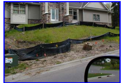
Silt Fence with Seeding
