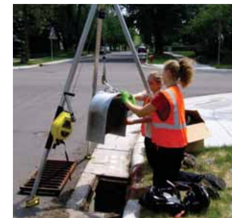
Staff maintains catch basins leading to the trench
