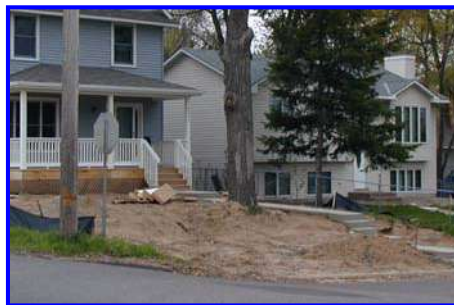
Residential Soil Erosion
