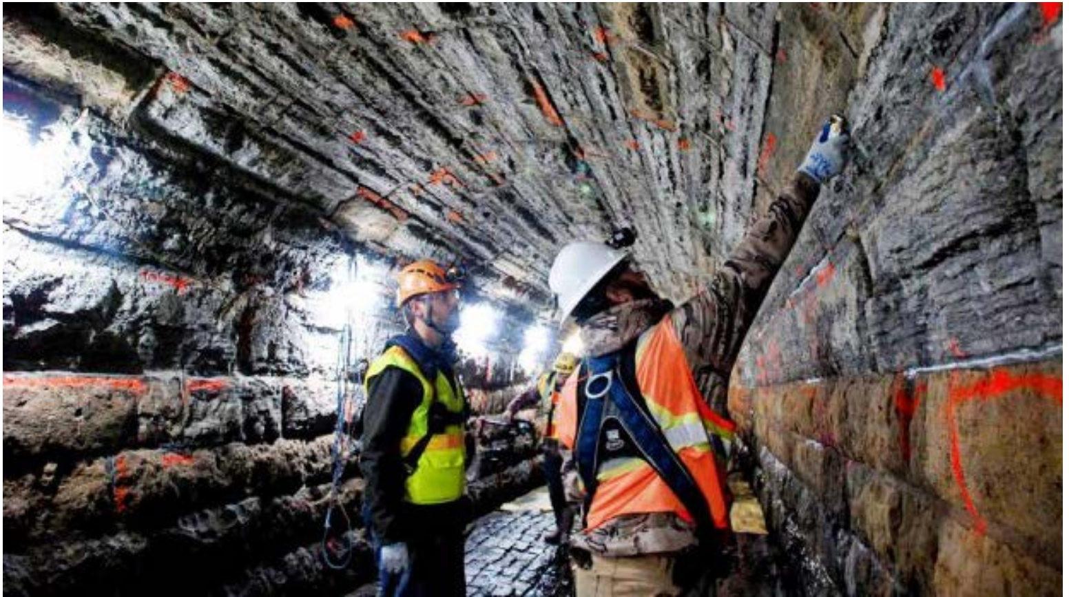
Workers with the Capitol Region Watershed District inspect mortar between the limestone blocks of the Trout Brook Storm Sewer system in St. Paul. (Courtesy of Capitol Region Watershed District)
