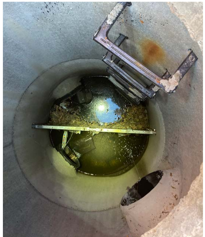
Inspection of permanent stormwater practices through the Permitted Sites Maintenance Program identified needed maintenance.
