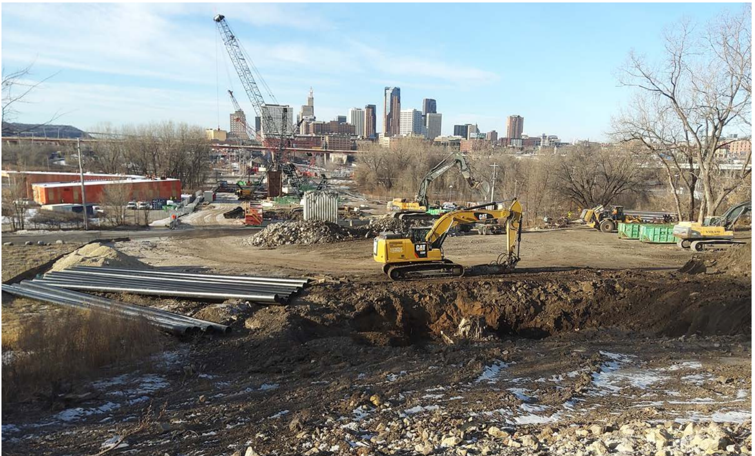
Active construction permitting work strives to keep soil and other materials contained within project limits and out of storm sewers and waterways.
